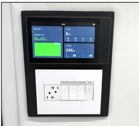
Power System Controller
