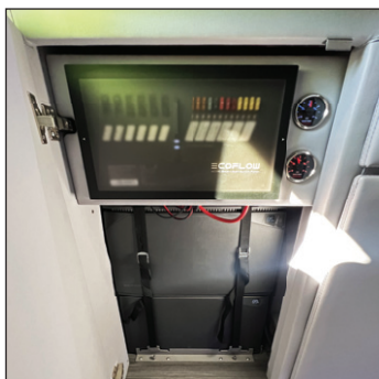
Power Hub & Batteries
