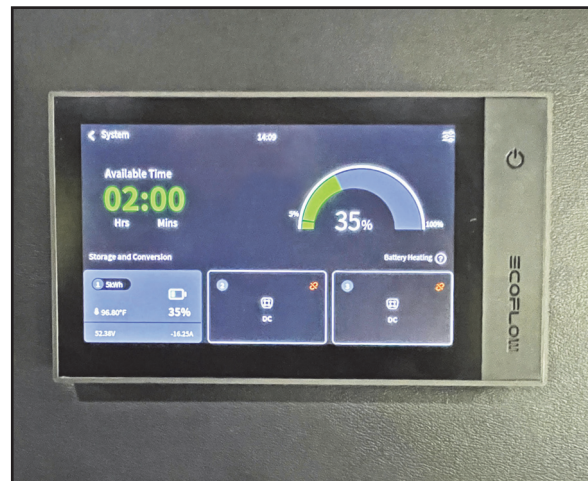
Power System Controller
