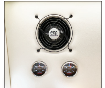
Tank Level Gauges
