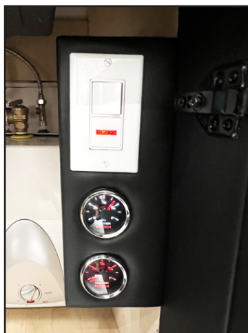
Water Tank Gauges
